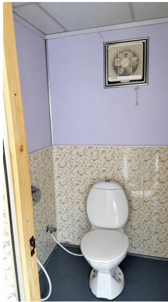
Prefabricated facilities portfolio | Compact sanitary fit-out within a modular facility
