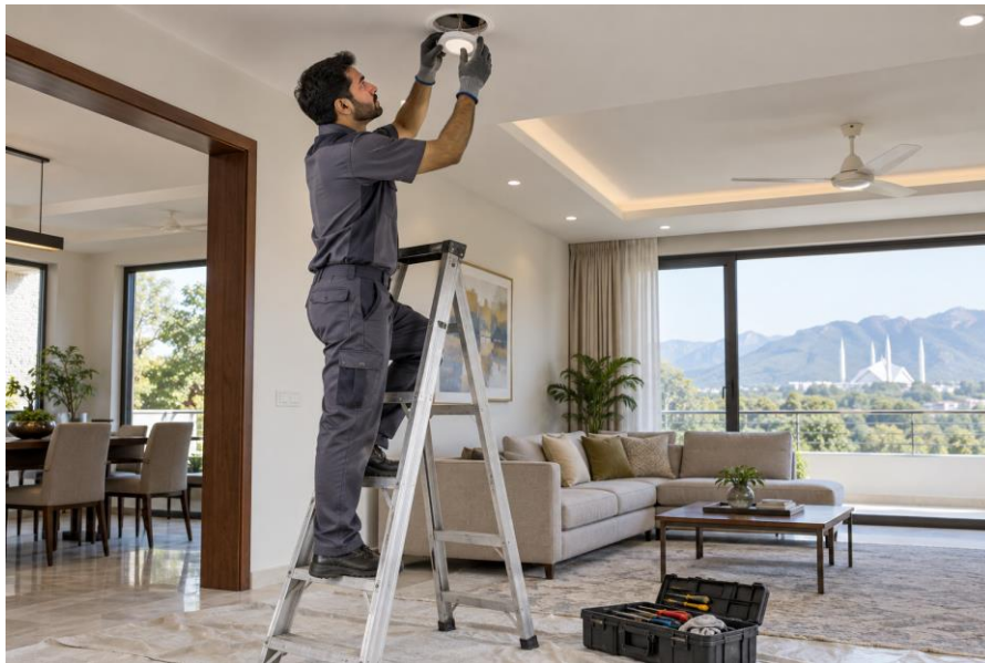
Illustrative service example | Ceiling and lighting maintenance
